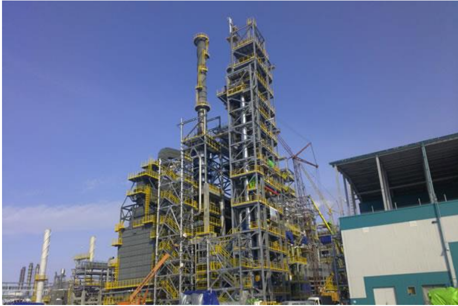
Figure 1 : Propane Dehydrogenation Unit (PDH) in Russia
